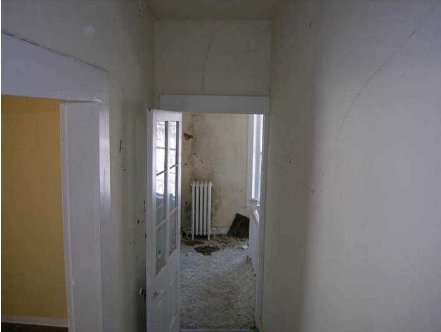
Upper level hallway, looking from the largest bedroom to the stairwell. The right side wall was added at a later point, and is the probable cause of structural stress in the main floor living room ceiling.
