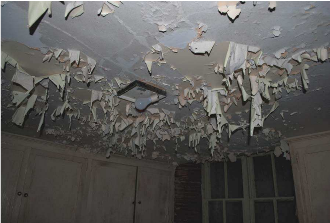
Figure 17. Moisture intrusion and its effects on paint and plaster in the lower level kitchen (see lower level floor plan for photo vantage point).
