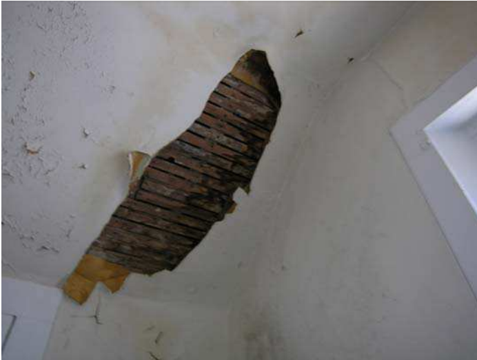
Water damage in upstairs bedroom ceiling
