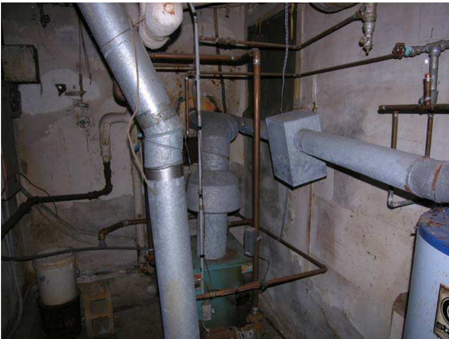
Lower level utility room
