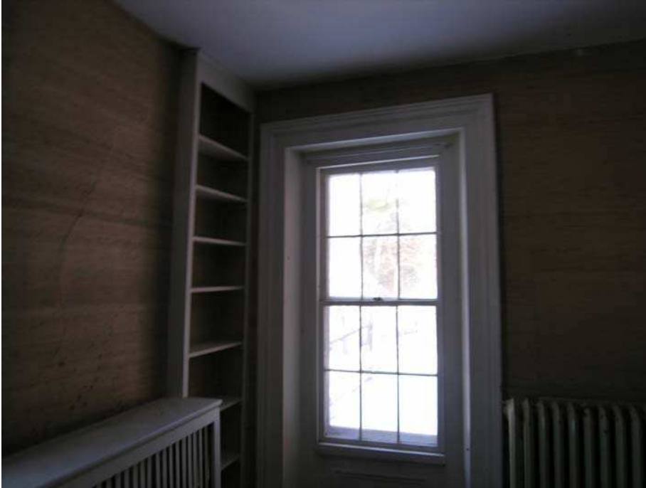
Northeast corner of main floor bedroom. This corner appears to have moved, or is moving.
