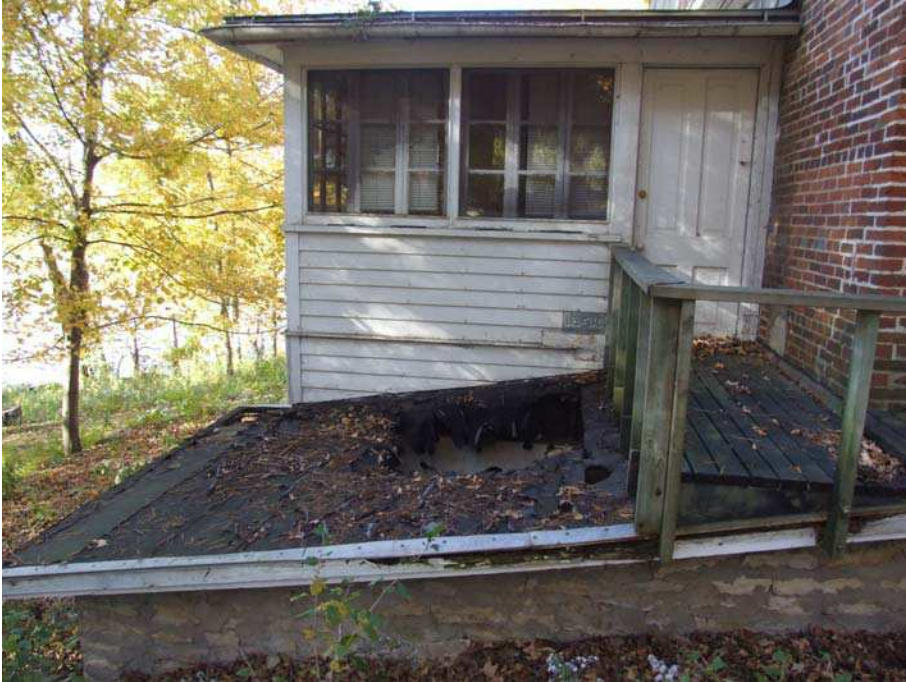
Figure 16. Collapsed roof on cellar (see lower level floor plan for photo vantage point).
