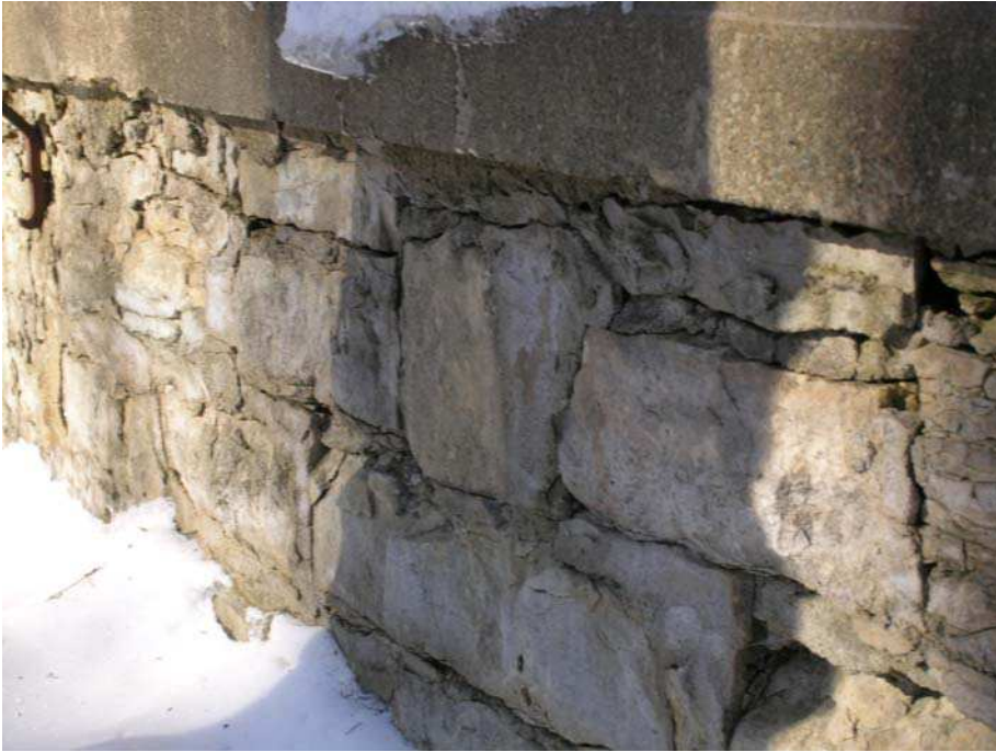
Crumbling limestone foundation under concrete terrace
