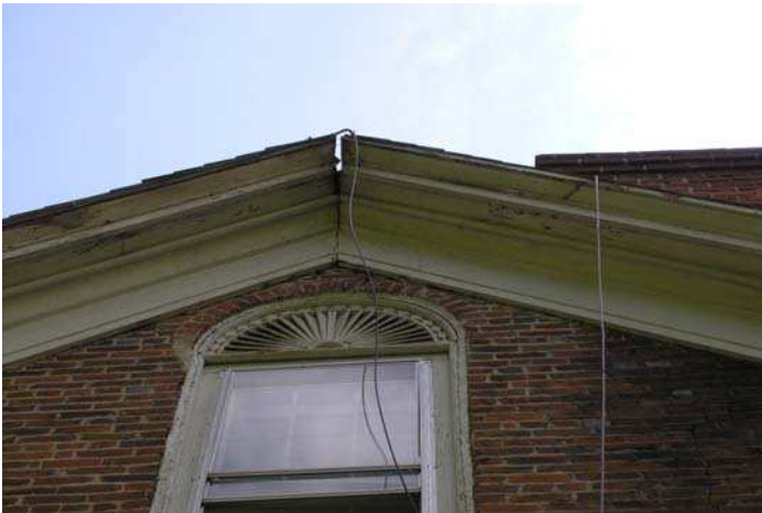
Exterior gable detail, showing trim separation. Some of the cracking and shifting appears to have been caused by settling. Crack monitors need to be installed and monitored to understand whether the cracks are active.
