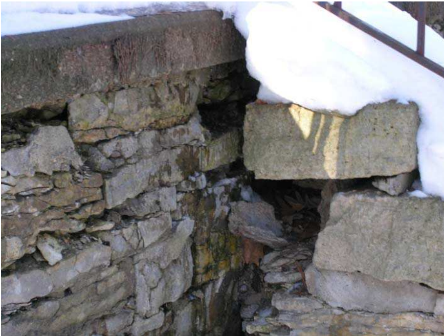
Crumbling front steps and foundation
