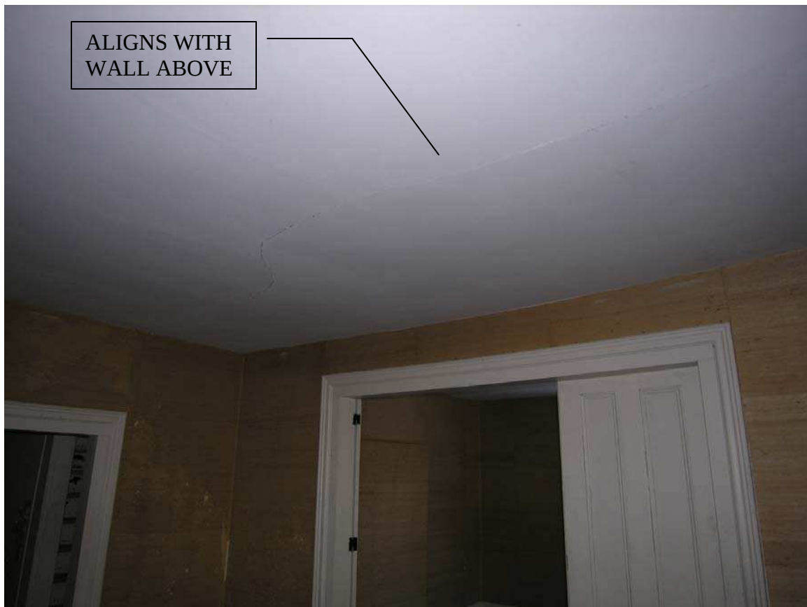
Main floor living room showing cracked plaster and sag in ceiling. The wall above, probably added during remodeling, unduly transfers the roof load to joists in the floor/ceiling assembly.
