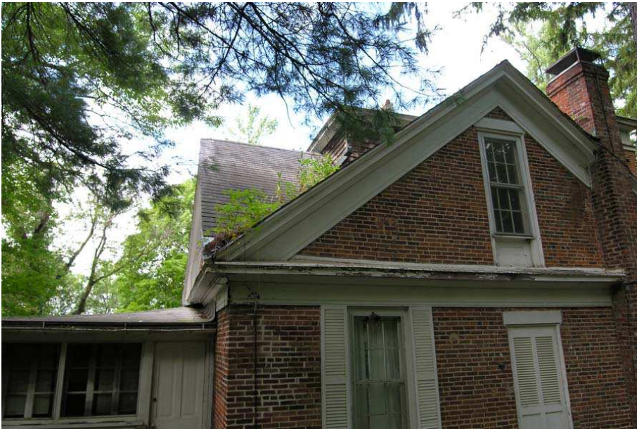
Small tree growing out of gable roof
